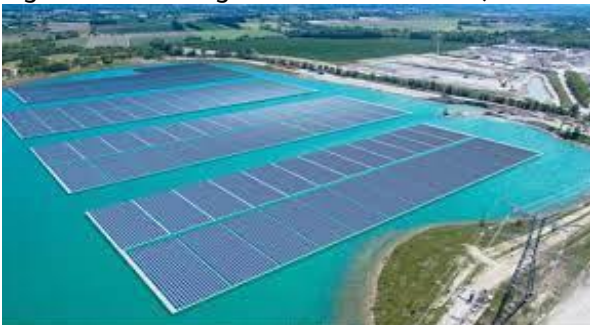
Figure 1.1: Floating solar PV installation (Source: Offshore Engineer)
